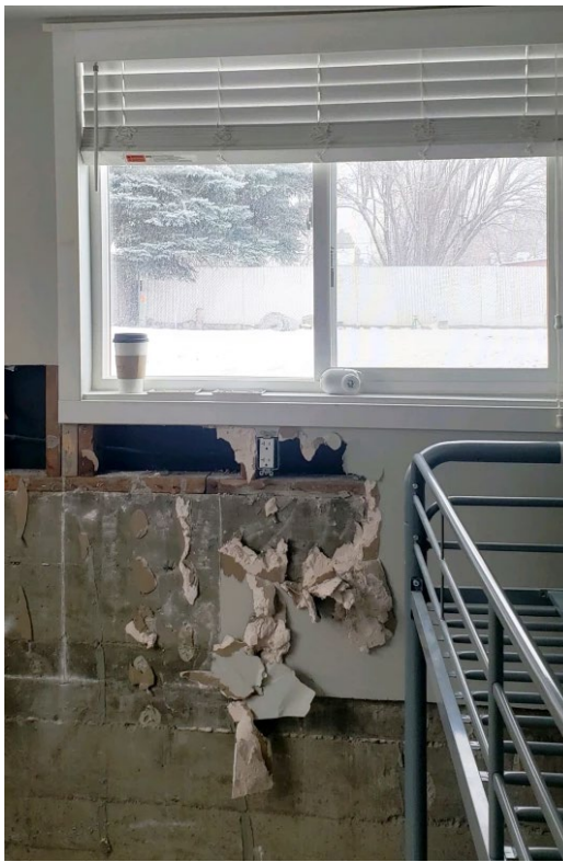
Drywall was removed and mold was discovered in the home of Alec and Taryn Wright.
